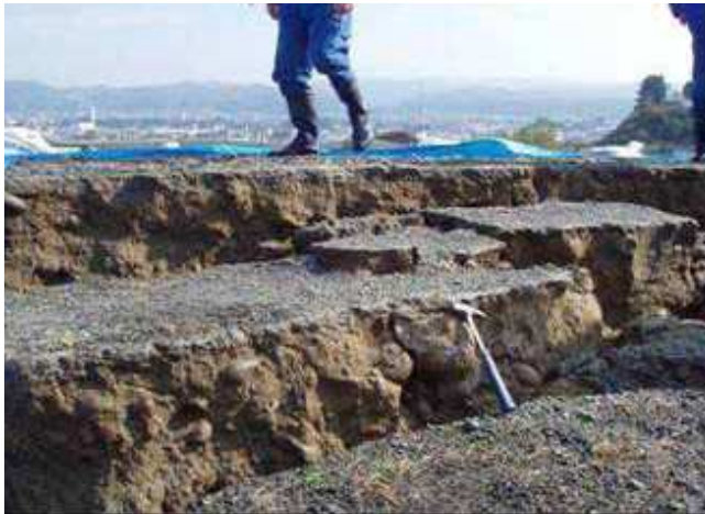
Stepping caused by crest cracking (Asagawara Regulating Reservoir)
