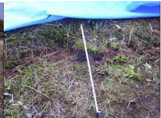
Crack on downstream slope (Tsuboyama Dam)
