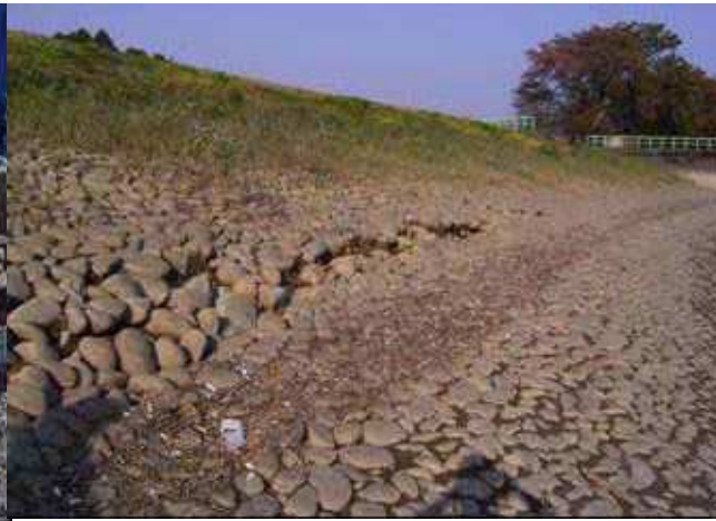
Slip of reservoir side slope (Yamamoto Regulating Reservoir)
