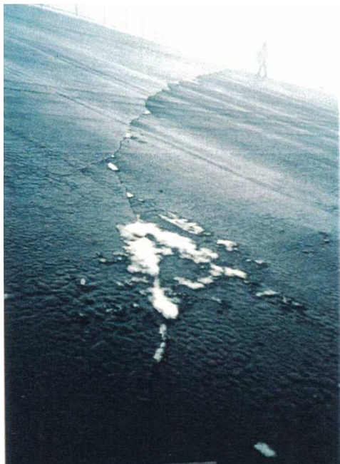
Cracks of Asphalt-facing discovered
